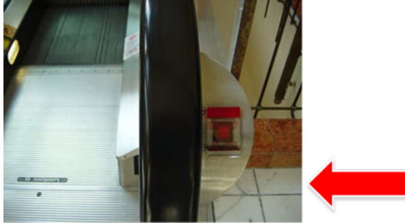
Figure 43. Emergency shut-off for escalator.
