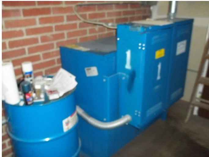
Figure 16. Example of a hydraulic pump and hydraulic fluid reservoir.
