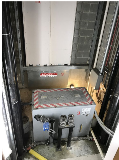
Figure 19. Hydraulic reservoir in the elevator pit of an MRL elevator.
