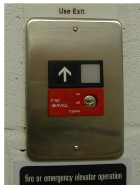
Figure 25. Lobby-level controls for initiating Phase 1 ERS.
