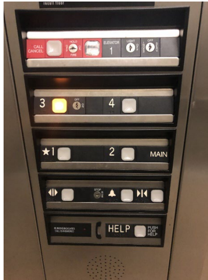
Figure 21. Controls within the elevator car.
