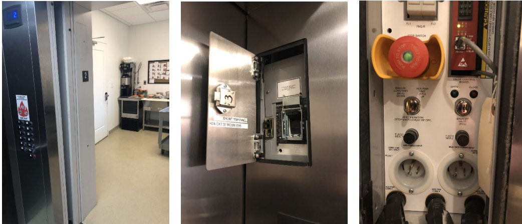
Figure 18. Example of elevator controls located within the elevator control space.
