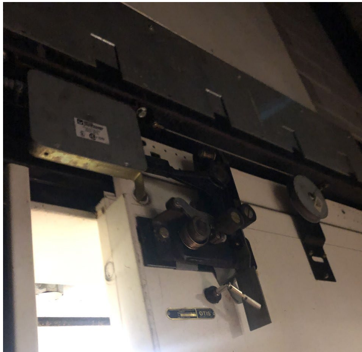
Figure 33. Hoistway key gaining access to hoistway by overcoming door interlock.
