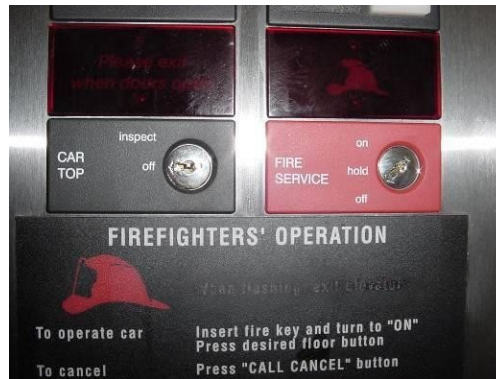
Figure 26. Interior elevator car controls used to initiate Phase 2 ERS.
