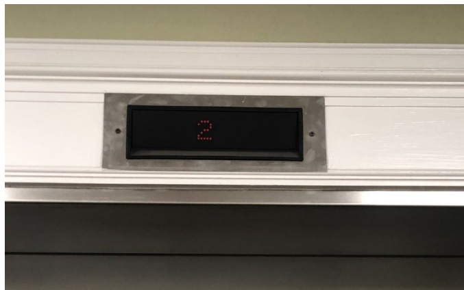
Figure 28. Floor indicator located in the lobby.
