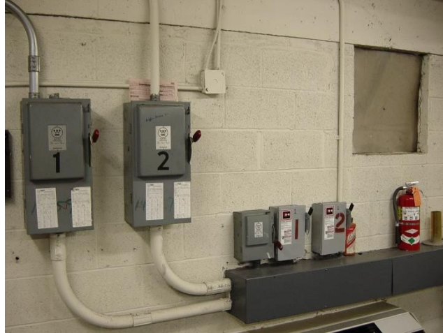
Figure 31. Two sets of electrical shut-offs for two elevators. The large disconnect boxes marked 1 and 2 on left are the mainline disconnects, and the small disconnect boxes marked 1 and 2 on right are the auxiliary electric shut-offs.
