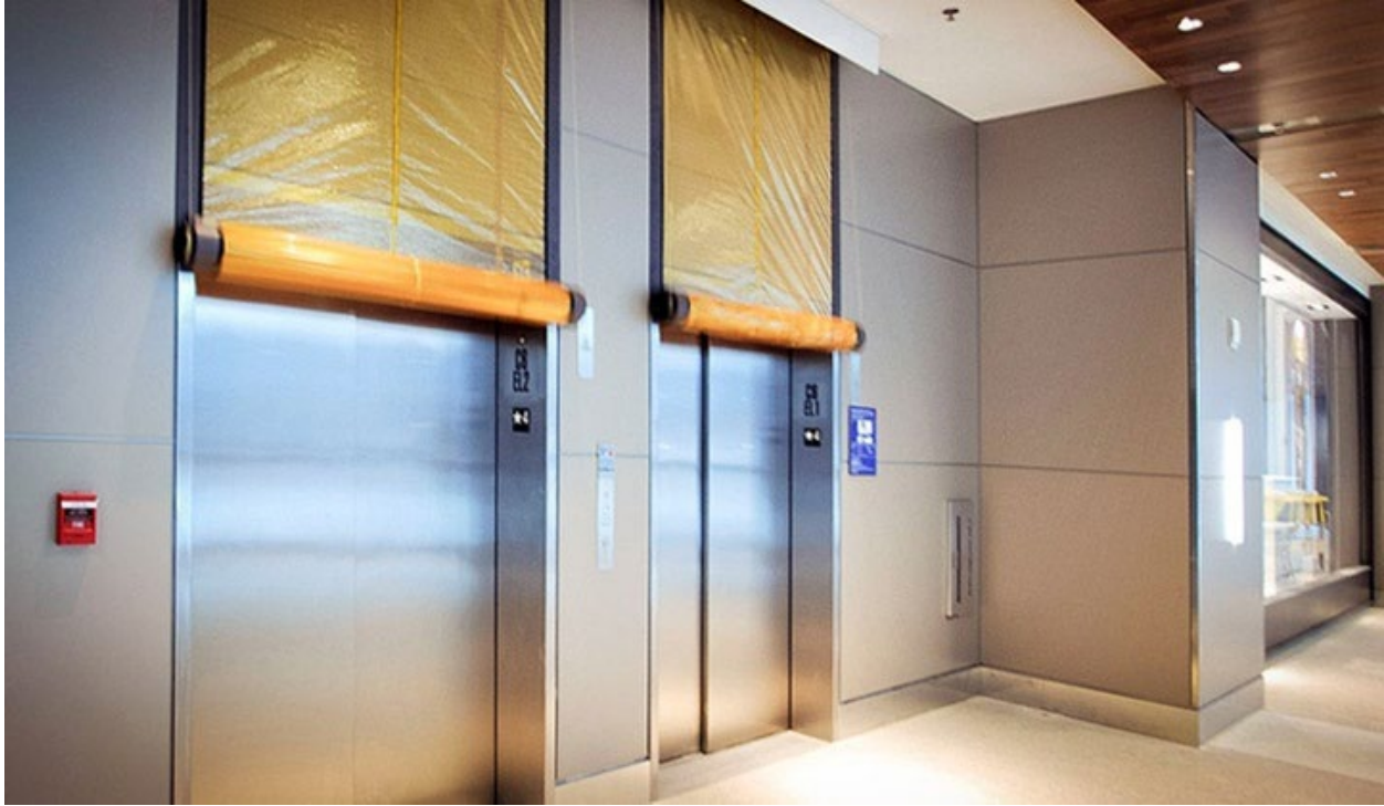
Figure 23. Elevator smoke curtain device activation.
