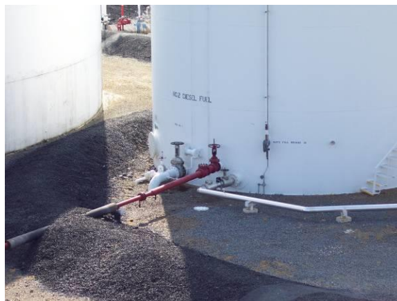
Figure 16: Red piping showing foam piped to sub-surface foam system.
