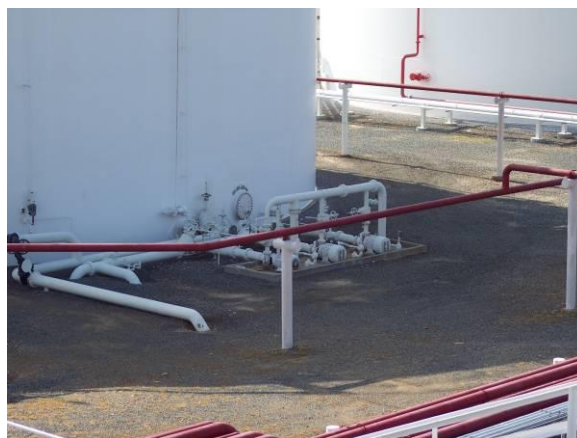
Figure 15: Fuel pumps in dike area.
