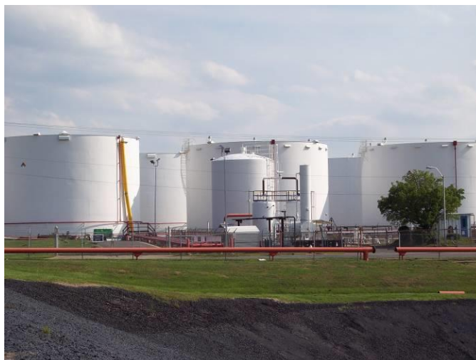
Figure 13: Bulk storage facility tank farm.
