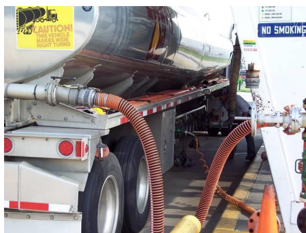
Figure 12: Loading rack with vapor recovery, electrical ground, and fuel fill hose attached.
