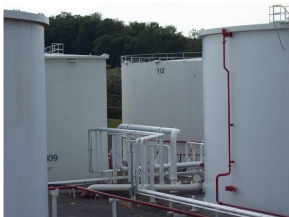
Figure 14: Flammable liquid piping in bulk storage facility.
