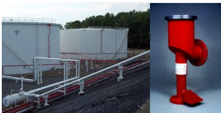
Figure 18: Fixed and semi-fixed foam protection systems designated by red piping. The figure on the right is a type II foam chamber.
