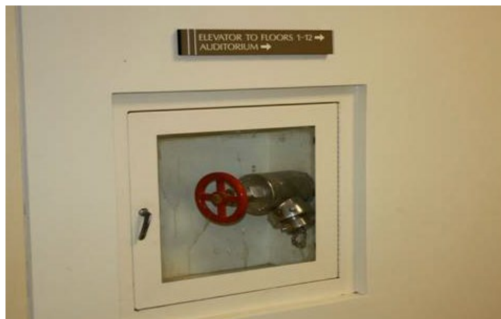
Figure 25. Standpipe riser outlet located in hallway midpoint.
