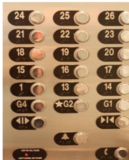
Figure 30. Blind shaft elevator control panel. Note lack of call buttons for Floors 2–12.
