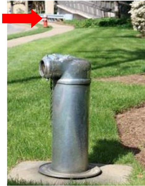
Figure 22. Hydrant located within 100 feet of FDC.
