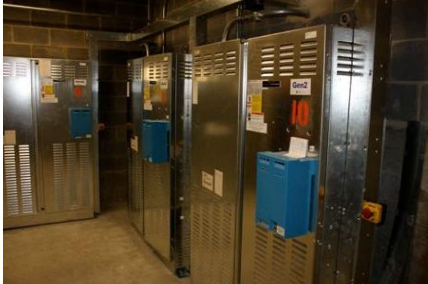
Figure 29. Otis Gen2 elevator.
