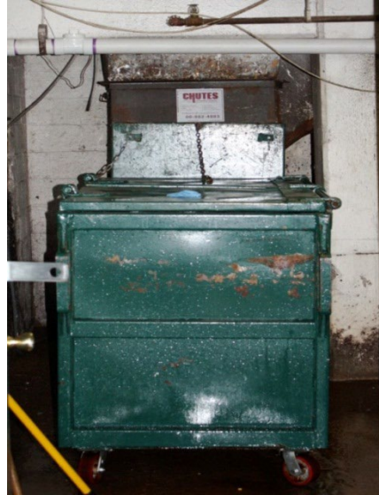
Figure 36. Trash chute and roll-out dumpster.
