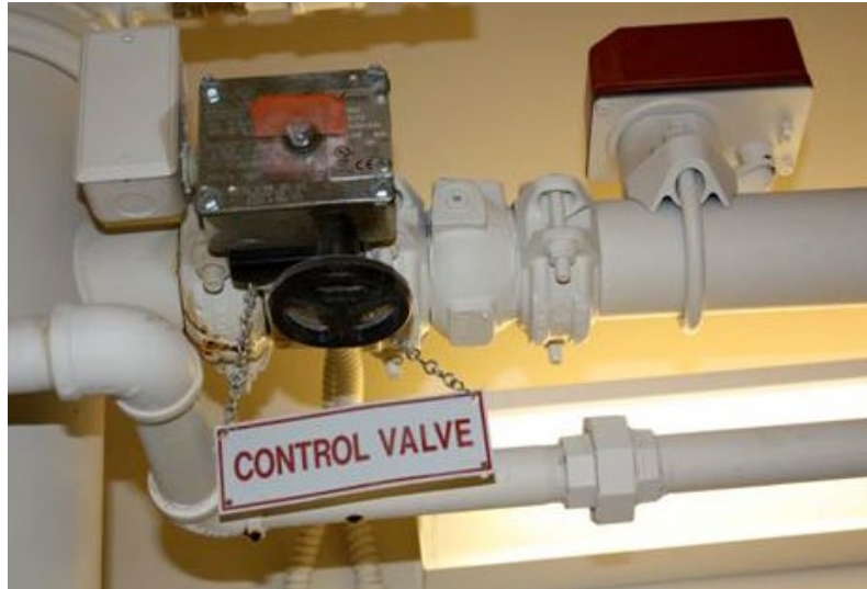
Figure 26. Sprinkler control valves.
