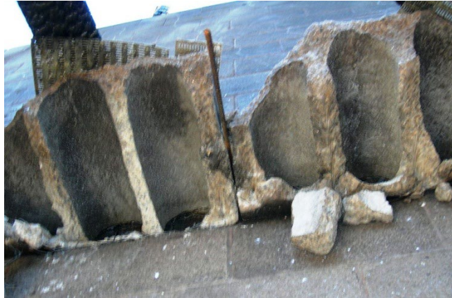
Figure 13. Failed lightweight concrete.
