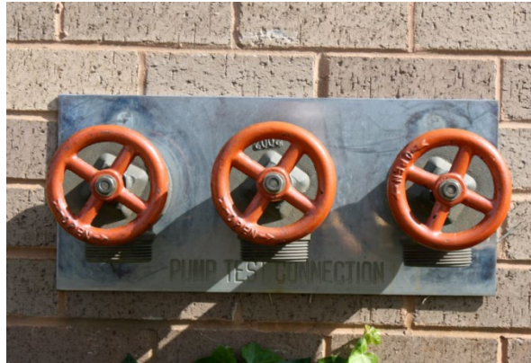
Figure 40. Test connections. These should NOT be used by fire department personnel.
