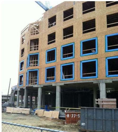
Figure 43. Podium construction used to build a lightweight, residential midrise over a noncombustible parking garage.
