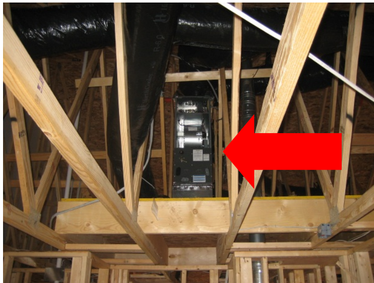
Figure 57: HVAC Unit in the Attic
