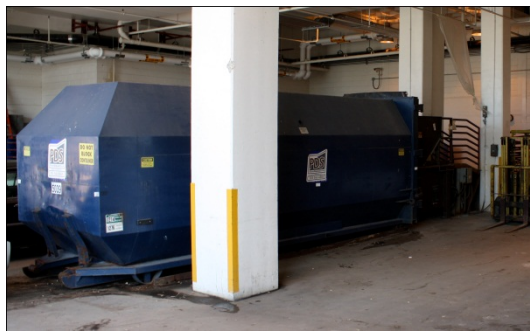
Figure 59: Many Trash Chutes Exit into a Dumpster or Compactor
