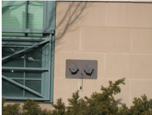
Figure 74: Supply all FDC Connections
