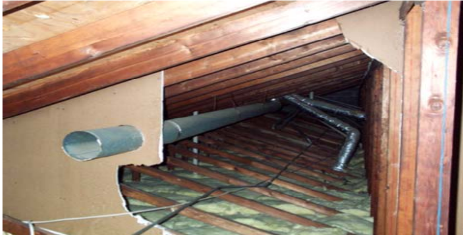
Figure 37: Breached Draft Stop
