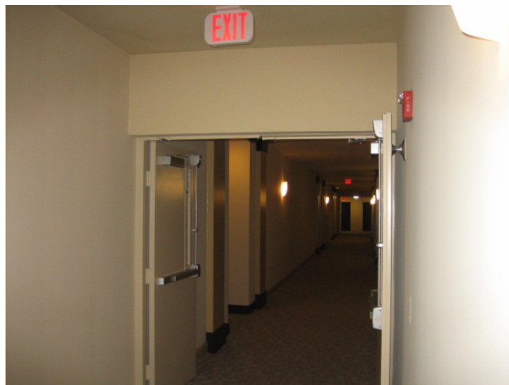
Figure 13: Example of Fire Doors
