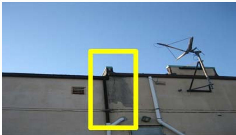
Figure 21: The Masonry Firewall that Extends above the Roofline Affords the Greatest Protection
