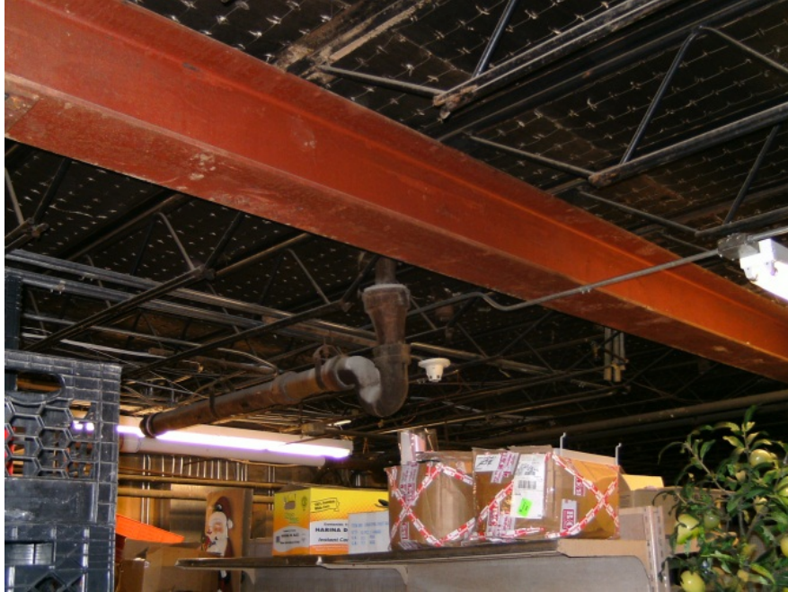
Figure 32: Note Significant Collapse Hazards in Building Preplans
