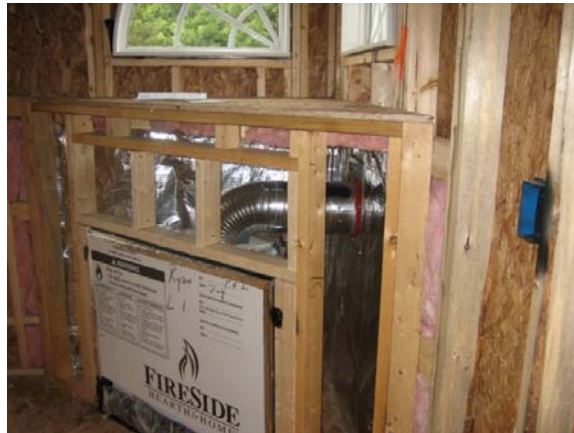
Figure 51: Zero-clearance Chimneys Create Potential for Fire Extension
