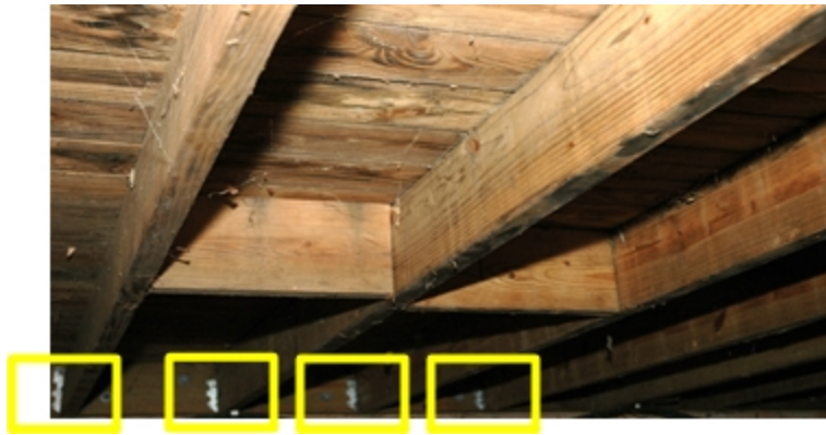
Figure 22: The Mass of Dimensional Lumber Provides Moderate Resistance to Collapse but Keep in Mind that the Metal Joist Hanger (Shown Outlined) is the Weakest Point
