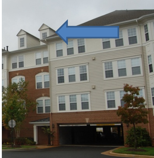
Figure 39: Companies should inspect Dormer Windows while Conducting Building Familiarization to Determine if they are Cosmetic or Indicate Living Space
