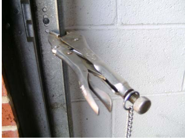
Figure 70: Securing an Overhead Door Using Vice Grips Placed High on the Track
