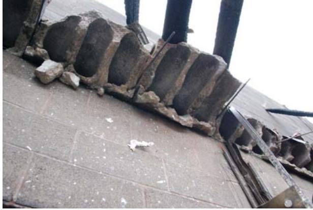
Figure 56: Lightweight, Non-combustible Concrete Floor that Collapsed Early in a Fire (View from Below)
