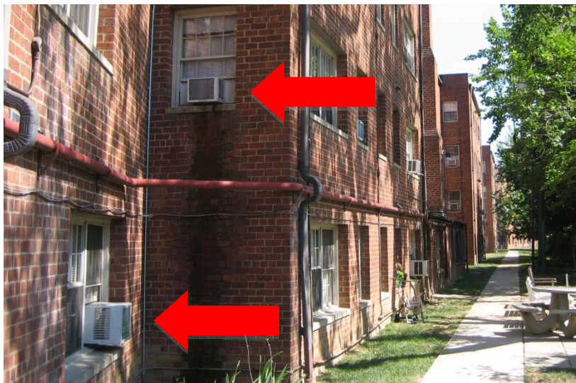
Figure 25: Window Air Conditioning Units are Common in 1940s-era Residential Buildings
