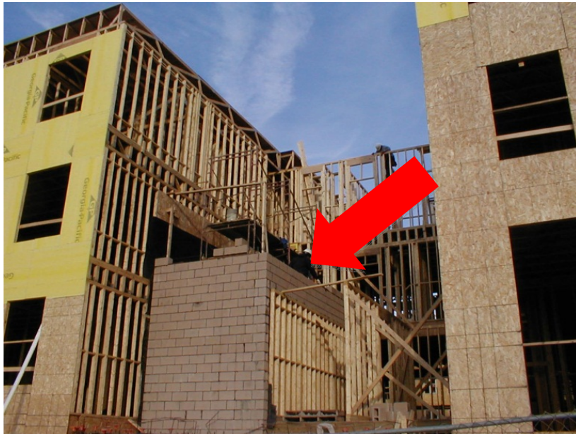
Figure 46: The Stairway is One of the Strongest Portions of the Lightweight Building
