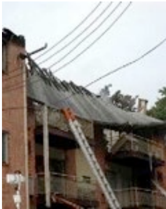
Figure 26. Attic overhang (i.e., soffit) collapse.
