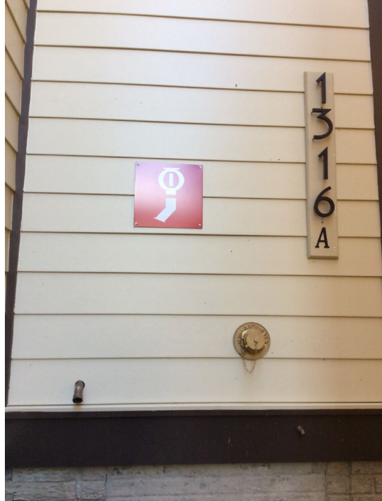
Figure 19. Typical fire department connection on a townhouse
