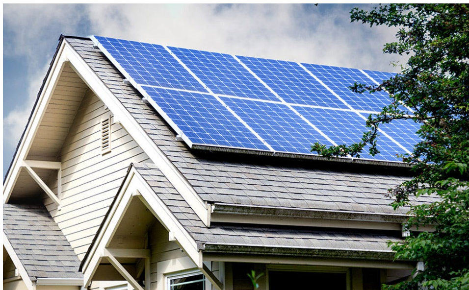
Figure 11. Solar panels installed on residential shingled roof.
