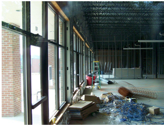
Figure 8. Lack of fire stopping between occupancies.
