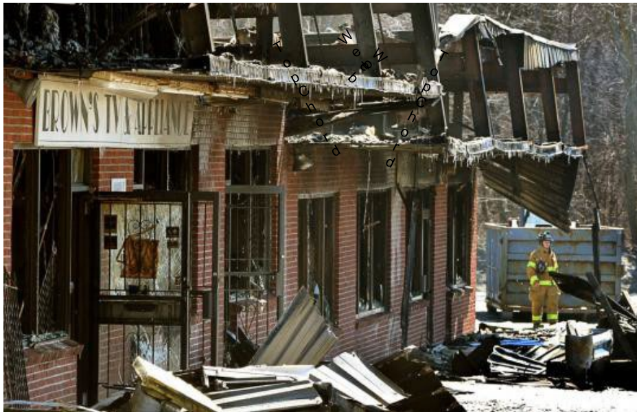
Figure 23. Fire spread to facade with collapse in a strip shopping center fire in Northborough, Massachusetts.
