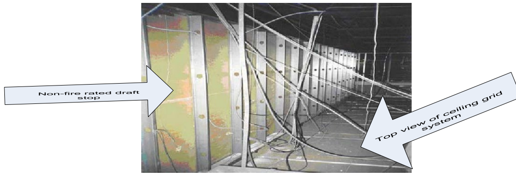
Figure 9. Non-fire-rated draft stops made of gypsum or plywood impede horizontal fire movement.
