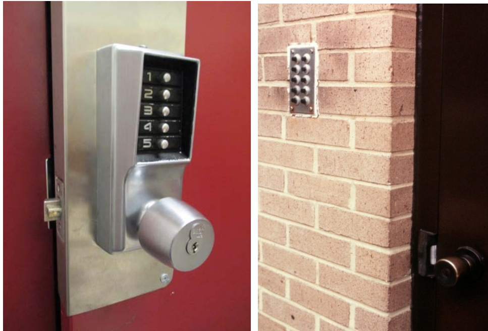
Figure 31: Cypher lock/knob combination (left) and electronic lock installed in the wall (right).
