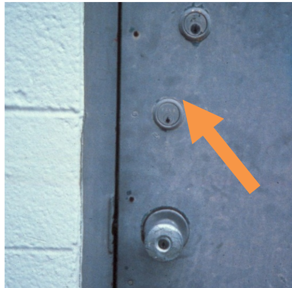
Figure 4: The absence of key marks and/or painted over lock face can identify a non-operational lock.
