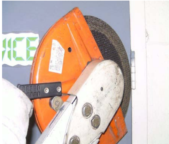
Figure 50: Using a metal composite-type blade to cut the hinges off a door.
