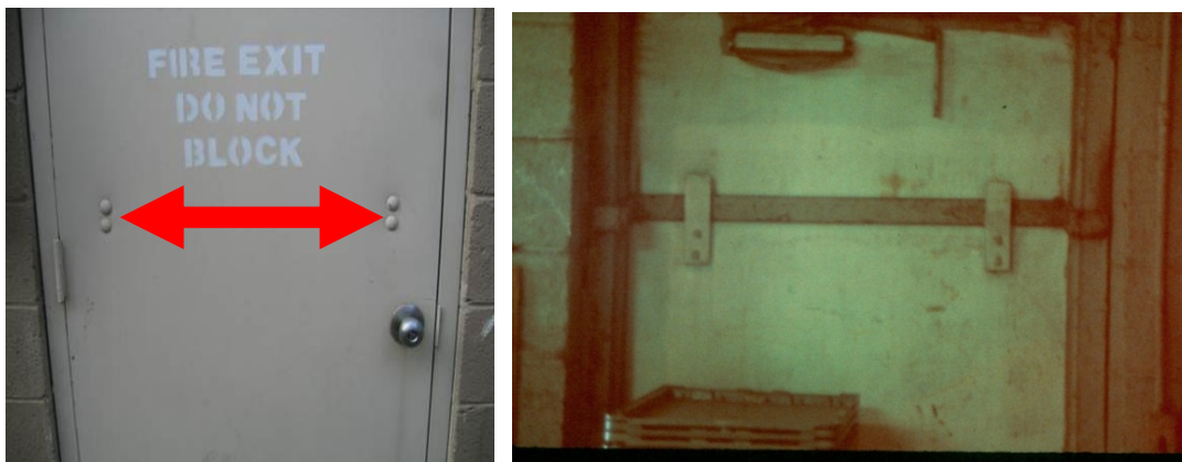
Figure 54: The presence of bolt heads can signify the presence of a drop bar.
