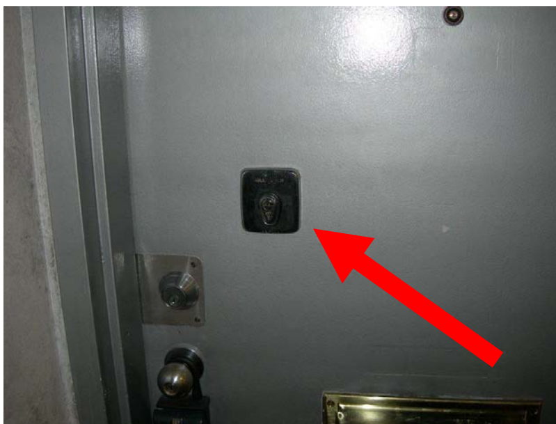
Figure 53: Exterior view of a multi-lock; use multiple hydraulic door opening tools at the top and both sides, then push the entire door inward.
