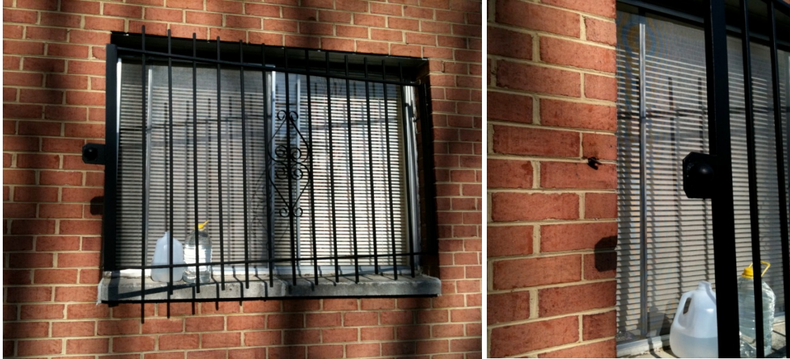
Figure 38: Some window bars are able to be opened and closed from within the occupancy.
