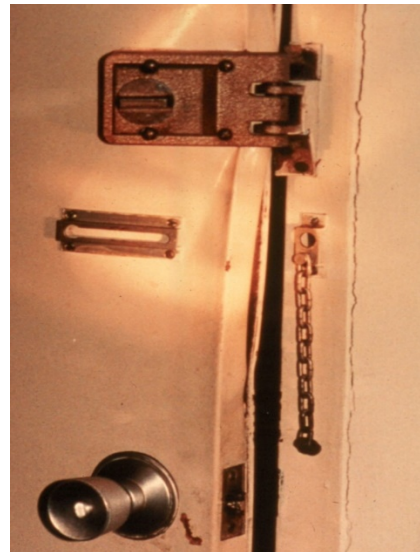
Figure 25: Door forced with a hydraulic forcible entry tool that was low on hydraulic fluid – tool failed to open the door because it lacked full power.
