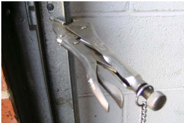
Figure 58: The primary method of securing an overhead door is to bend the tracks. If not feasible, placement of channel locks on this track is acceptable.
