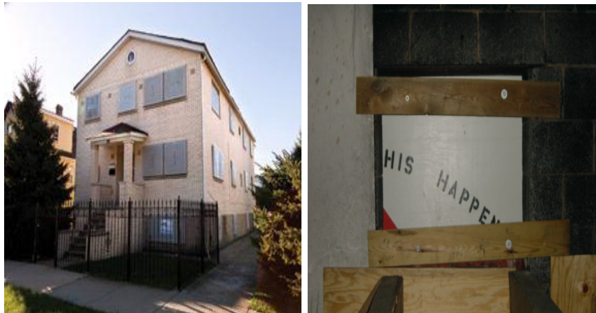
Figure 42: VPS manufactured window and makeshift HUD window.
