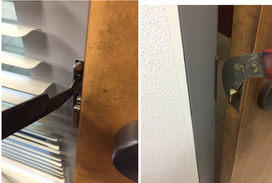
Figure 14: Shove knife used in door with a night latch (left) and used on a door without the dead latch (right).
