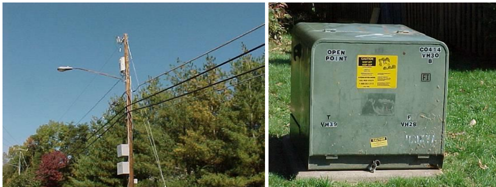
Figure 26: Examples of pole (left) and ground (right) transformers.
