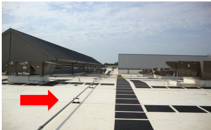
Figure 16: Rooftop commercial HVAC units and exposed gas lines.
