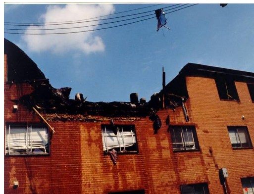
Figure 23: This apartment building exploded due to the storage of a propane tank on the third floor.
