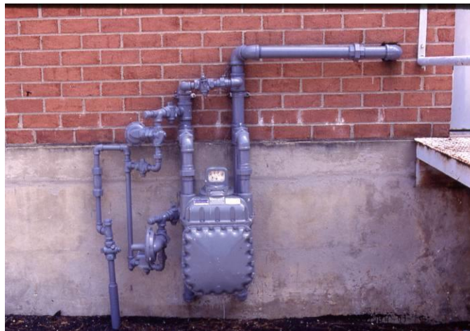
Figure 9: Commercial gas meter.
