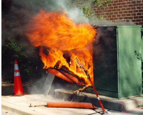
Figure 31: Ground transformer fire.
