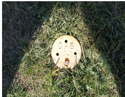
Figure 20: Curb box located in a yard.
