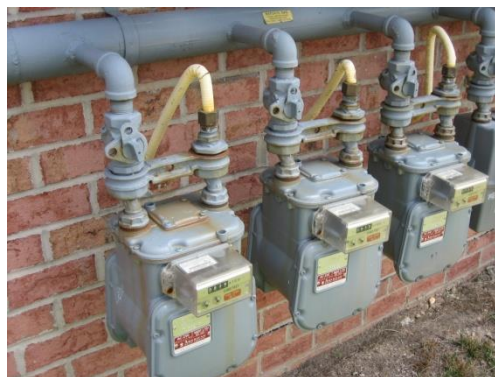
Figure 5: Gas main where flexible hose has been used.
