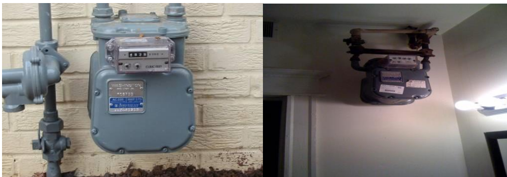
Figure 17: Two basic types of gas meters: outside (image on left) and inside (image on right).
