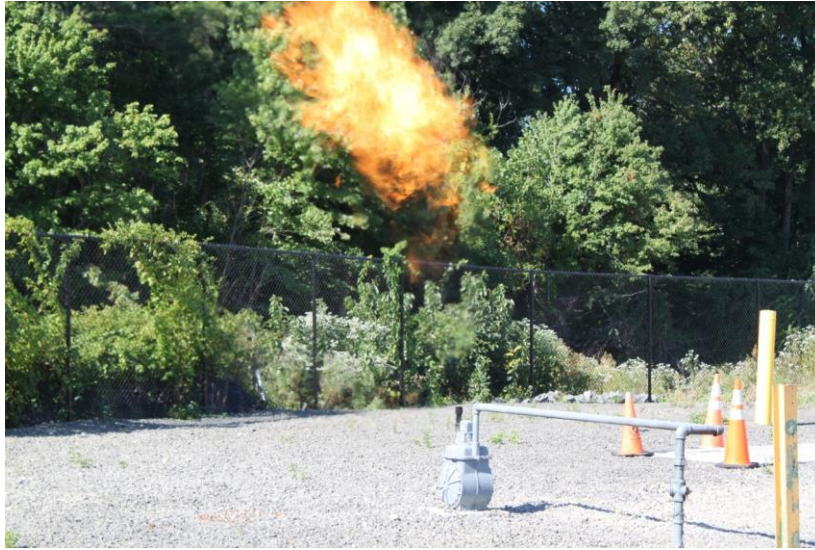
Figure 14: Fire involving the gas meter.
