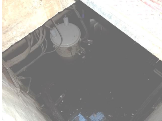
Figure 32: An underground electrical vault; they are commonly filled with water.
