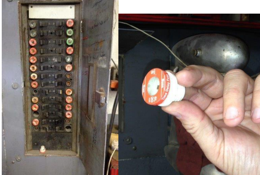
Figure 39: Older homes may still have screw-in fuse style panels.
