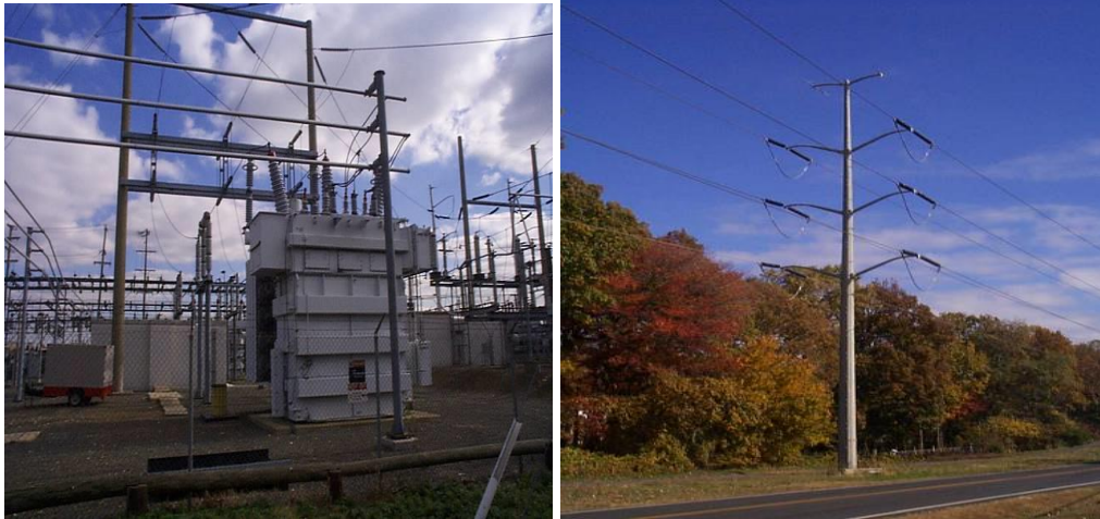
Figure 25: An electrical substation (left) and primary lines (right).
