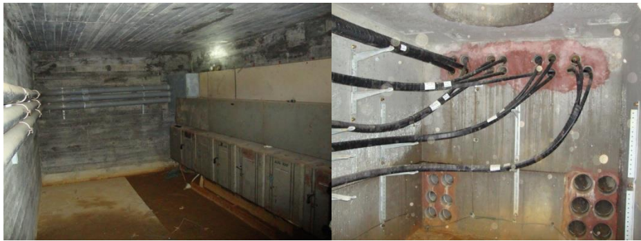
Figure 33: This figure shows an older underground electrical vault (left) and a newer one (right).
