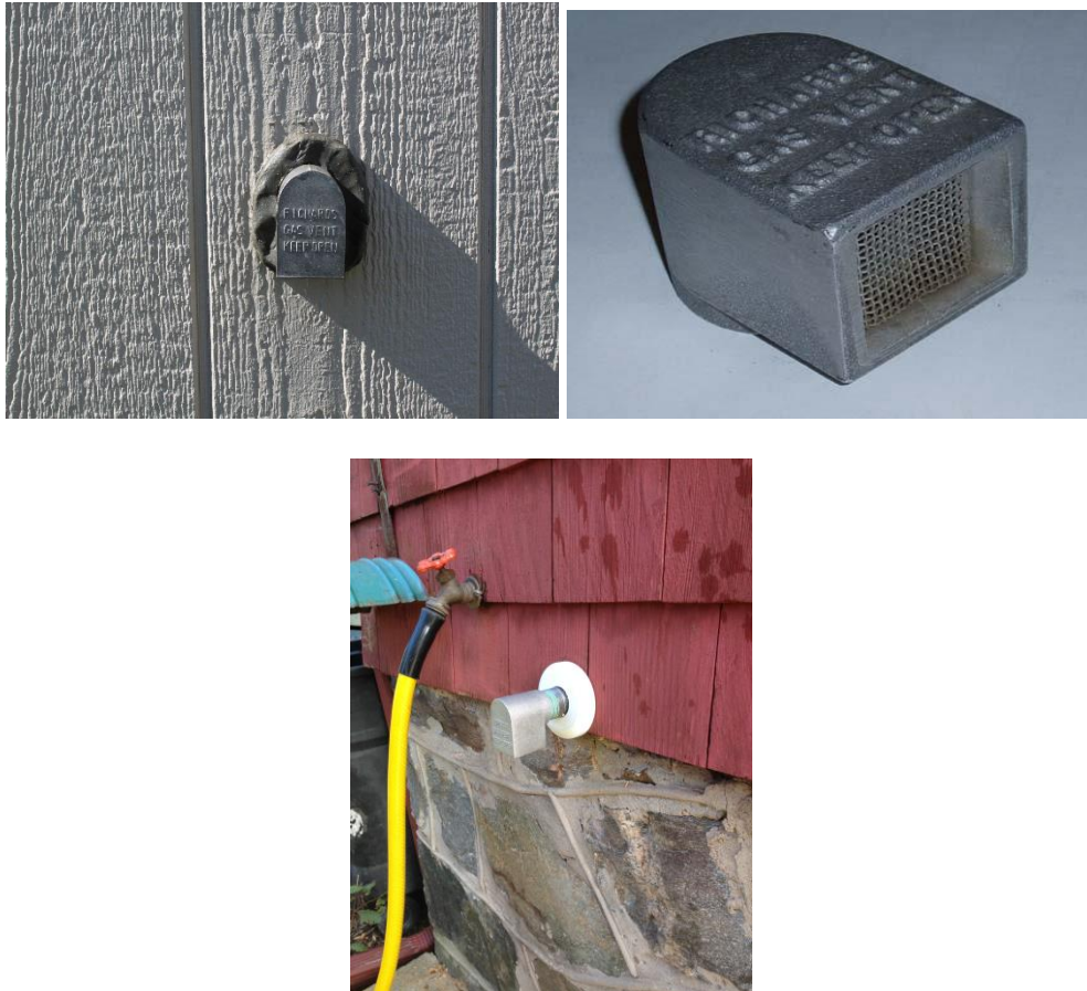
Figure 18: Examples of gas vents; the presence of a gas vent on an exterior wall is an indication of an inside gas meter.
