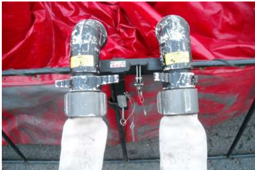
Figure 6: 3-inch Supply line holder.
